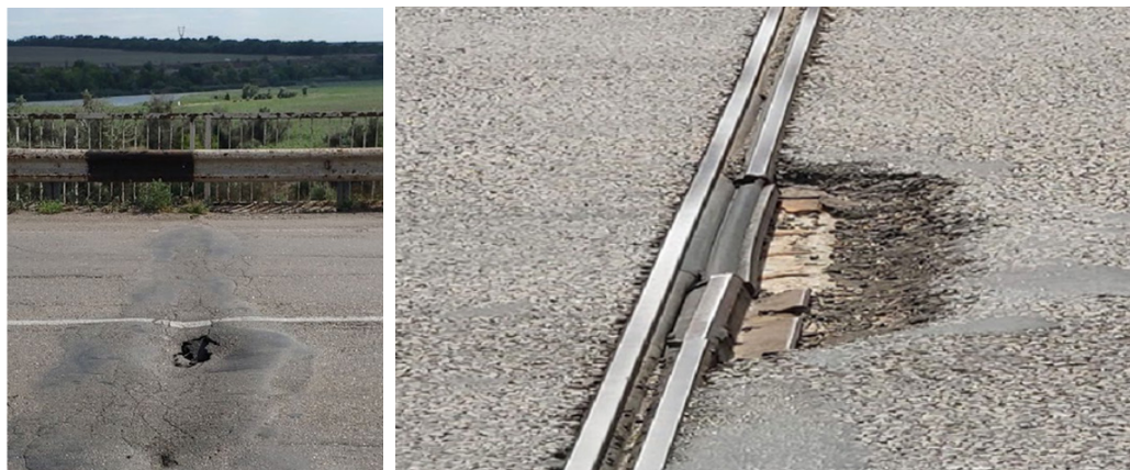
Fig. 5. Characteristic defects of bridge pavement in the area of expansion joints
